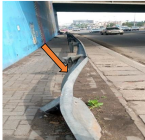
Figure. 23 Damaged and mangled crash barrier in poor condition at the TMI barrier at TQI
