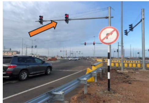
Figure 19: Traffic Signal at TMI
