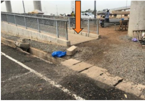
Figure 14: Entrance to a footbridge ramp at TMI with loose gravel and open drains gravel surface and open drains
