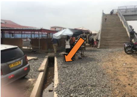
Figure 15: Access to a staircase at TMI with loose
