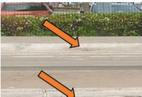
Figure 10: 42 cm high kerbs (arrowed)
