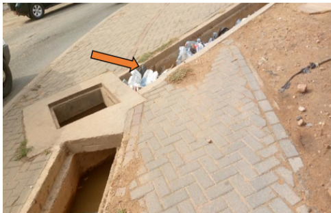
Figure 7: Walkway at TQI with open drains and uncovered manholes
