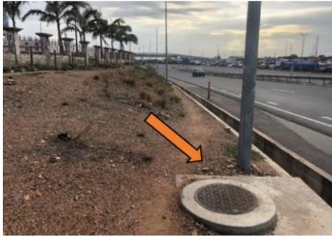
Figure 5: Walkway covered by manhole
