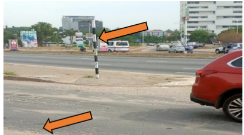
Figure 17: Damaged signpost and faded Pedestrian crossing (TQI)
