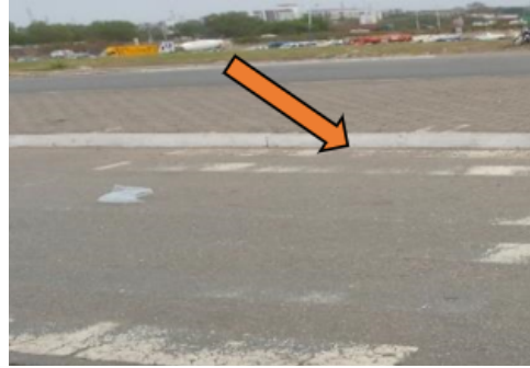
Figure 11: Kerb ramp on only one side of road pedestrian crossing at (TQI) with faded pedestrian crossing (TQI)
