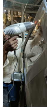
Fig 53: Using the heat gun to bend the fibre glass to conform to the shape of the door
