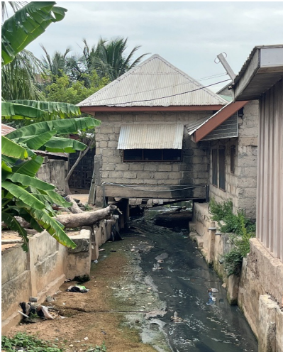
Plate 1: Unapproved extension to existing
