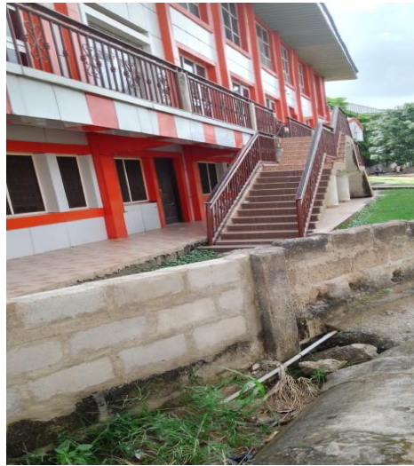
Figure3: A picture of a storey church building with a weak foundation blocking a waterway with a wall
