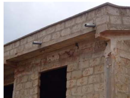
Plate 3: Example of the use of sandcrete blocks in constructing a parapet wall.
