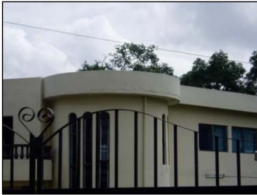
Plate 4: Shows a crack in the cement/sand plaster where the blockwork meets the concrete slab
