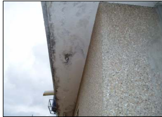
Plate 5: Discolourations due to seepage
