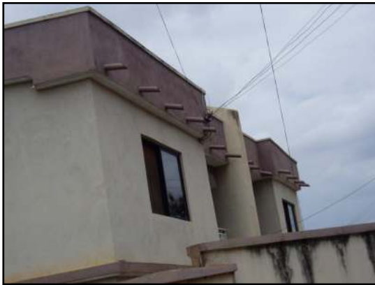
Plate 6: Shows the introduction of extra rain water spouts in the parapet walls of the roof to solve the problem of leakage.
